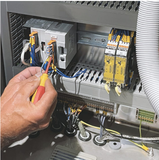
Service & Maintenance Reliable service that keeps you running without interruption.
